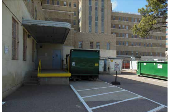
A service area behind Building 500 is located off 19th Avenue, separate from the main building entrance on Aurora Court.
