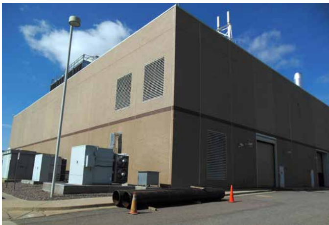
The CUP can accommodate boiler and generator expansions within the existing building envelope.
