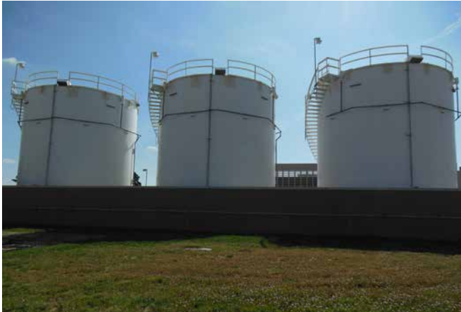
Fuel oil tanks located south of the CUP.
