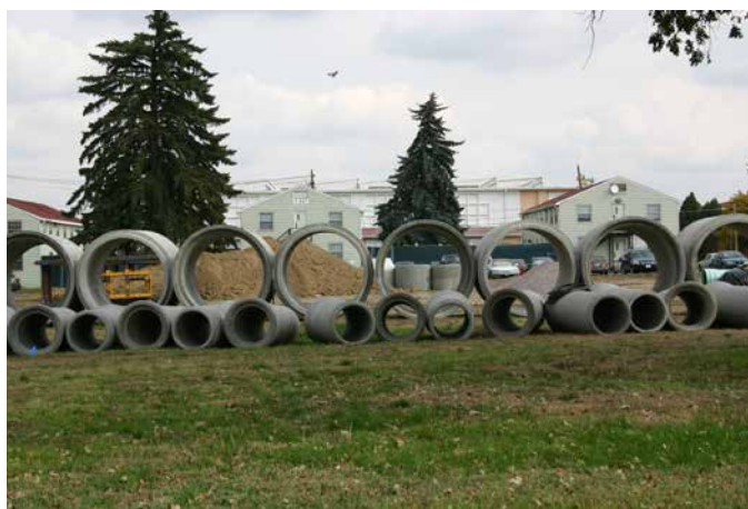
Pipes for the storm sewer system are laid out and ready to be installed.
