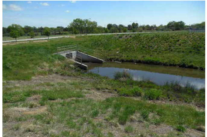
Water quality treatment infrastructure at Pond 374.
